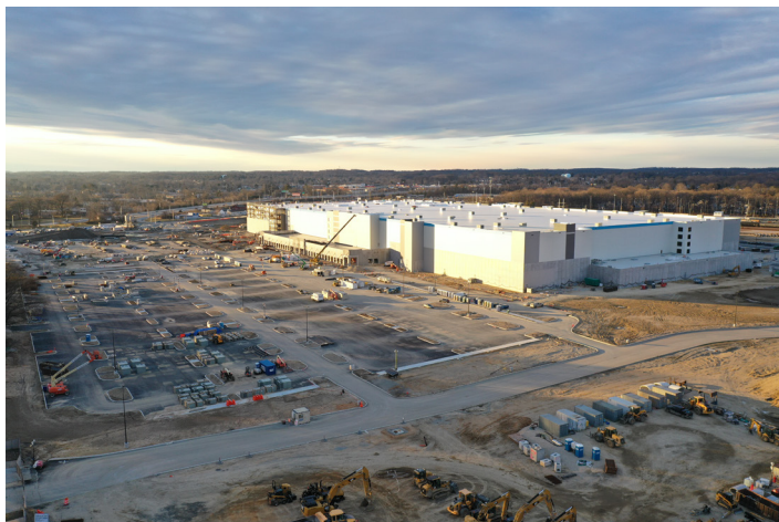
Courtesy of Dermody Properties , An Amazon fulfillment center under construction at the former site of General Motors' Wilmington Assembly on Boxwood Road in Wilmington, Delaware.
